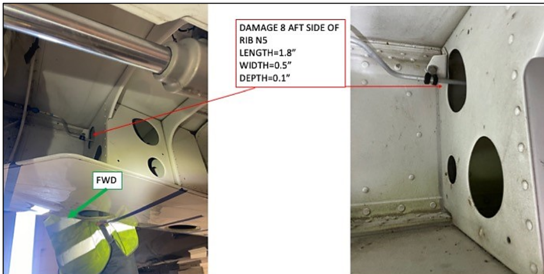
Figure 7. Damages to the left hand wing structure.
